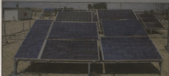
Photovoltaic array at the National Solar Energy Centre, Israel
